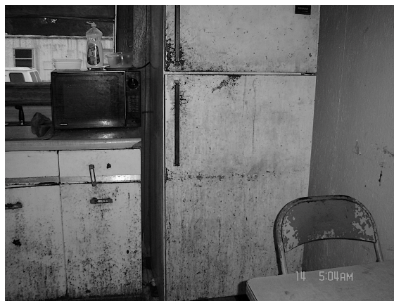
Figure 5: Moisture in the kitchen.
