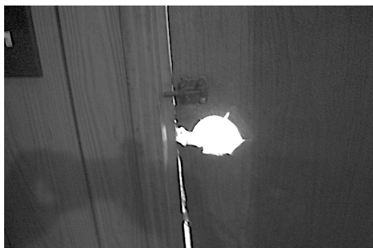
Figure 3: Security (broken locks and door knob).
